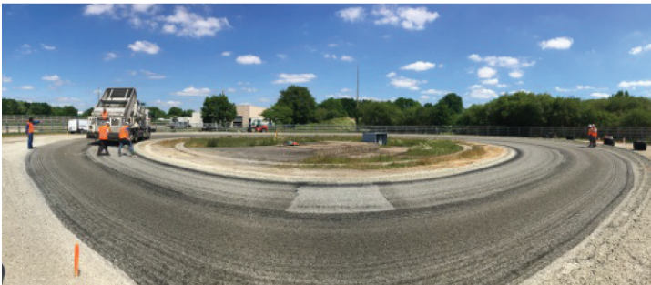
The pavement fatigue carousel
